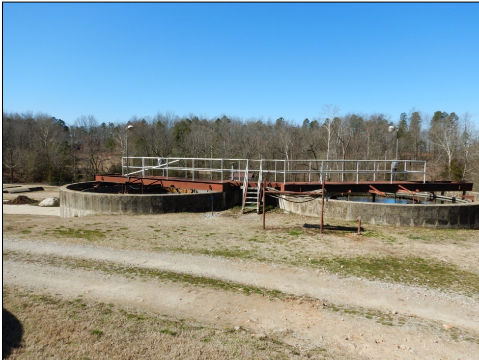
Photograph 4. Secondary clarifiers. The one on the left-hand side was out of service at the time of the site visit. The City rotates operation of the clarifiers for maintenance purposes.
