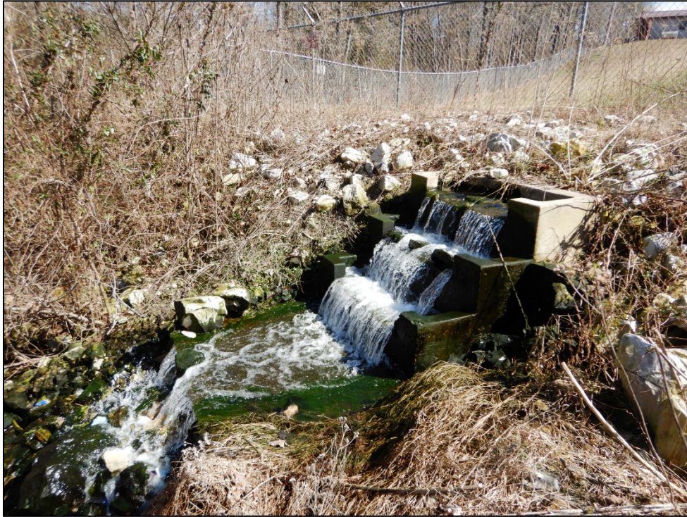
Photograph 9. Outfall and cascade post-aeration. A strong chlorine odor was present.
