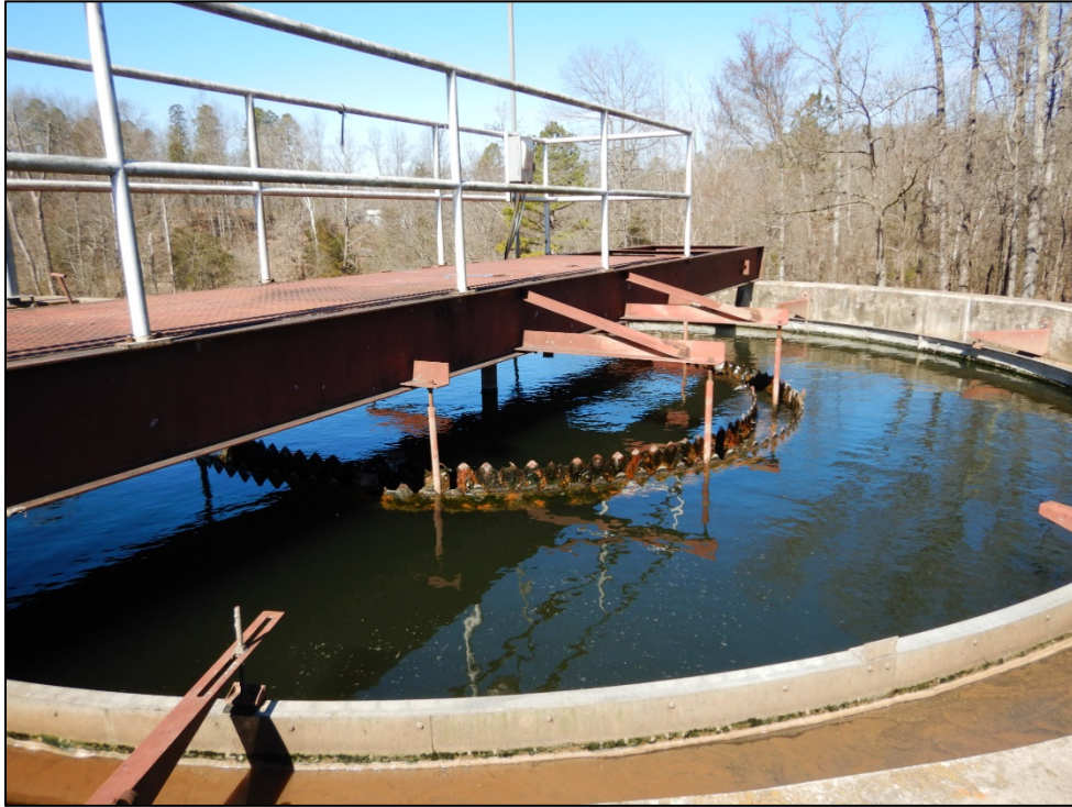
Photograph 5. Secondary clarifier (in service).
