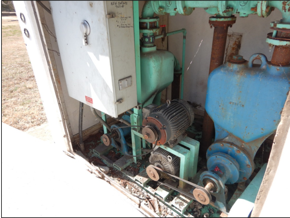
Photograph 11. Solids recirculation pumps. The drive belt for the motor on the left-hand side had fallen off during the site visit.
