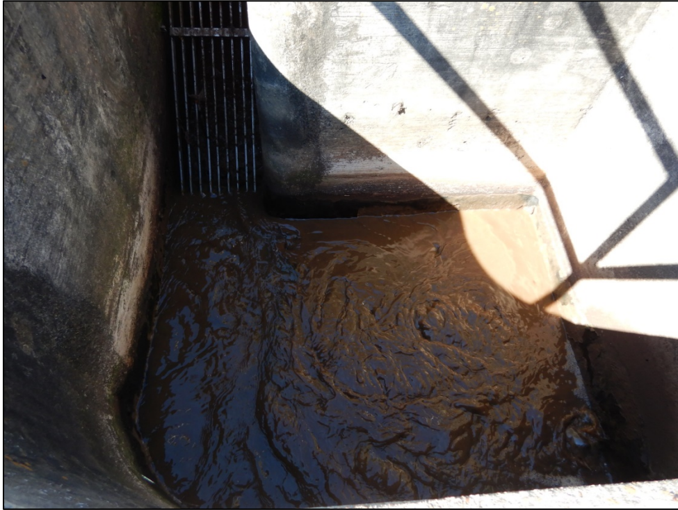
Photograph 1. Headworks influent channel and bar screen.
