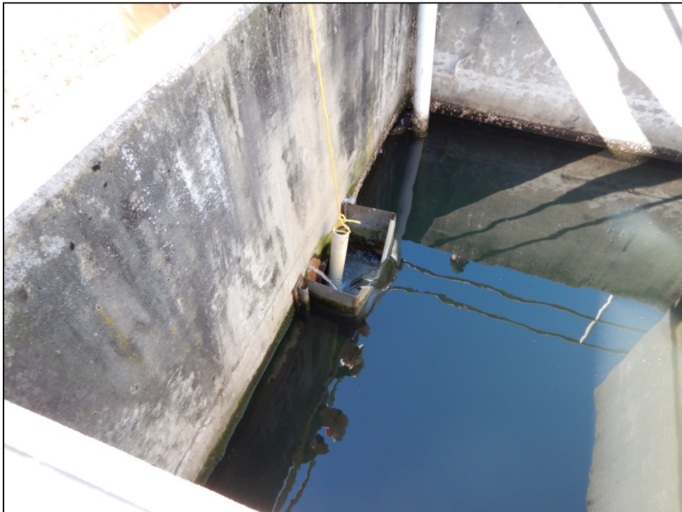
Photograph 8. Effluent end of the chlorine contact chamber. The hanging polyvinyl chloride pipe contains sodium sulfite tablets for dechlorination.
