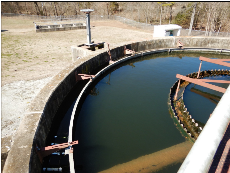
Photograph 6. Additional view of the secondary clarifier that was in service.
