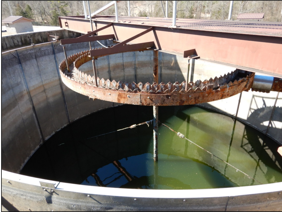
Photograph 7. The out of service secondary clarifier.
